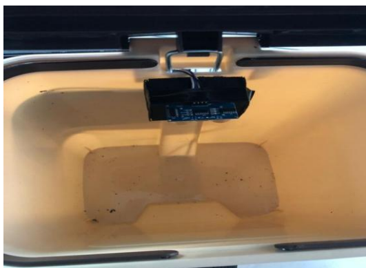
Fig. 3 Ultrasonic Sensor Installation
